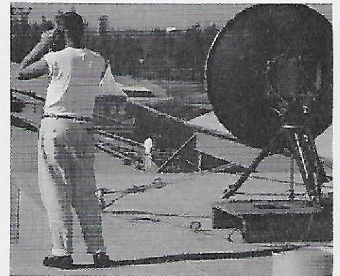
On roof, a micro-wave transmission link
