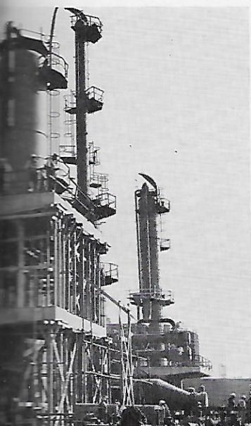
Nearing completion at Los Angeles Refinery are new Unifining and Platforming Units
